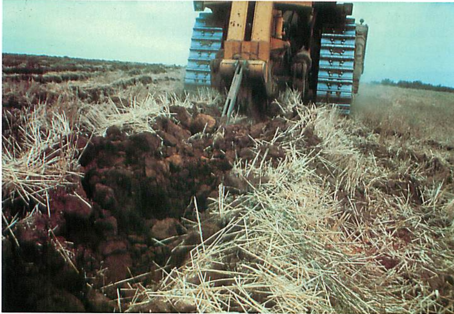
Figure 4.8. Deep ripping to a depth of 6 feet disrupts the upper 3 feet of soil.
